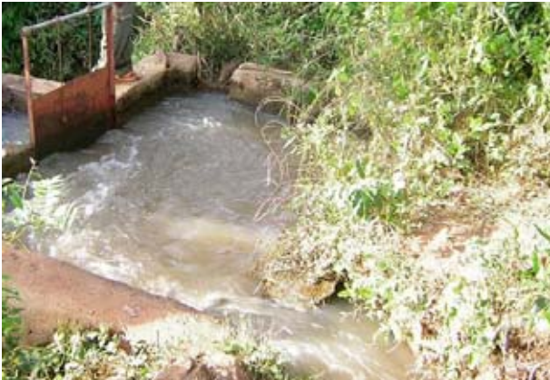
Water reservoir or also called forebay. From there the water flows through the penstock into the water turbine, by Dirk Hillerkus, 2009
