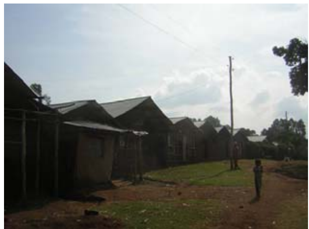
Electric poles provided and erracted with community participation and the btransmission line in the village of Bachani, Dano woreda, West Shoa zone. By Dirk Hillerkus, 2009.
